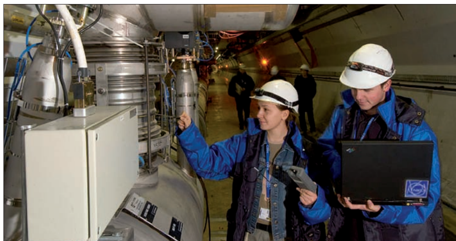
The first section of the LHC cryogenic distribution line, corresponding to an eighth of the accelerator, has been tested at a temperature of 10 K since the end of November 2005.
